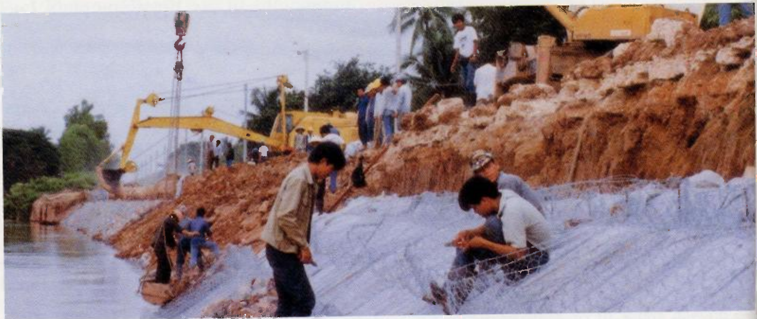
Rock-filled galvanized wire basket mattresses and retaining walls provide an excellent and durable means of bank integrity protection.
