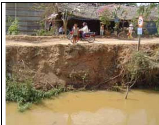
Figure 5.21 Sliding of PR855 after the 2007 flood.
