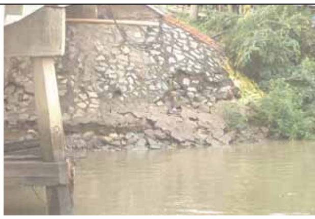
Figure 5.22 Damaged bridge abutment PR855.
