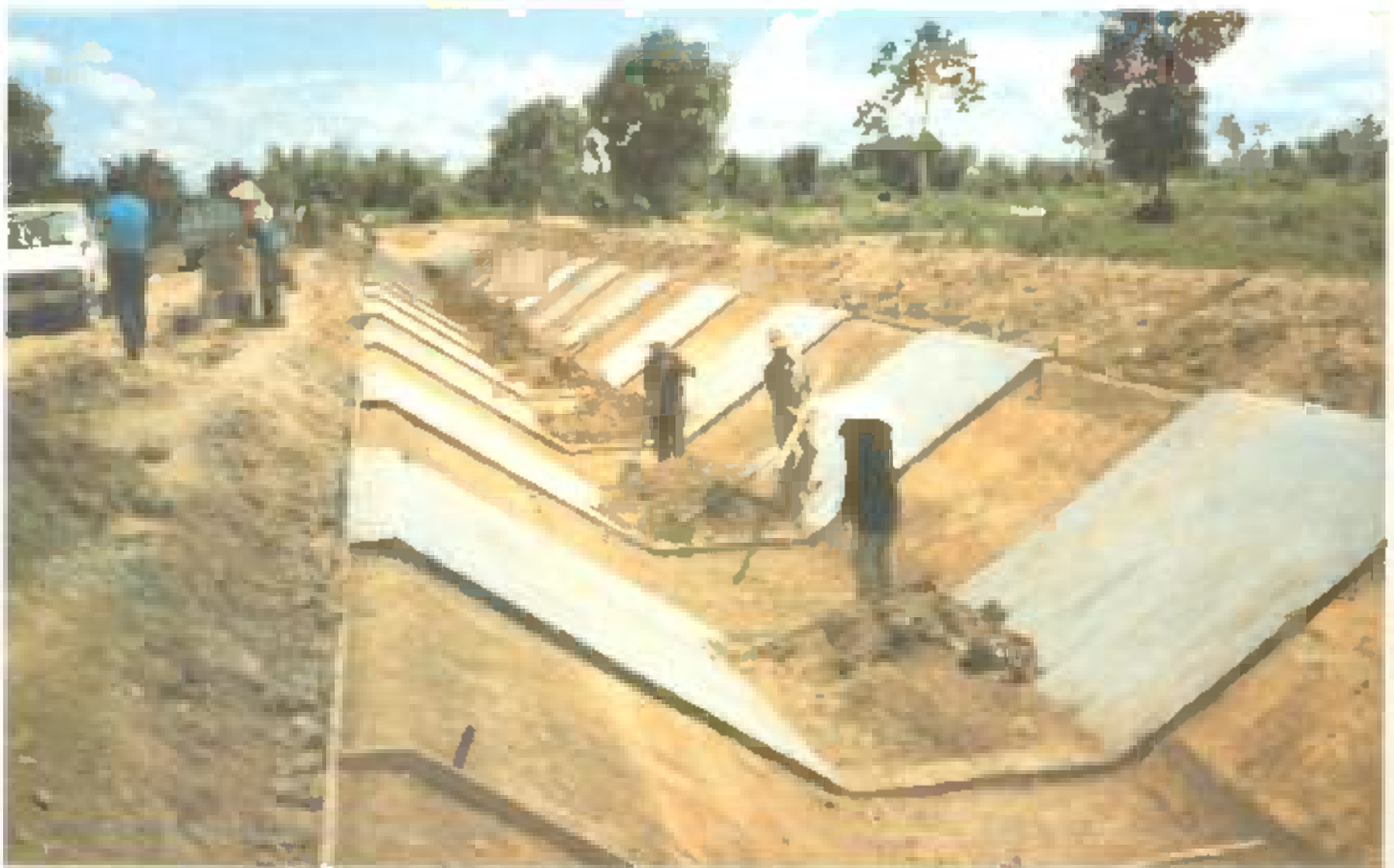
Preparation of the foundations for lining one of the main canals of the Huai Mong project, northeast Thailand, gets underway
