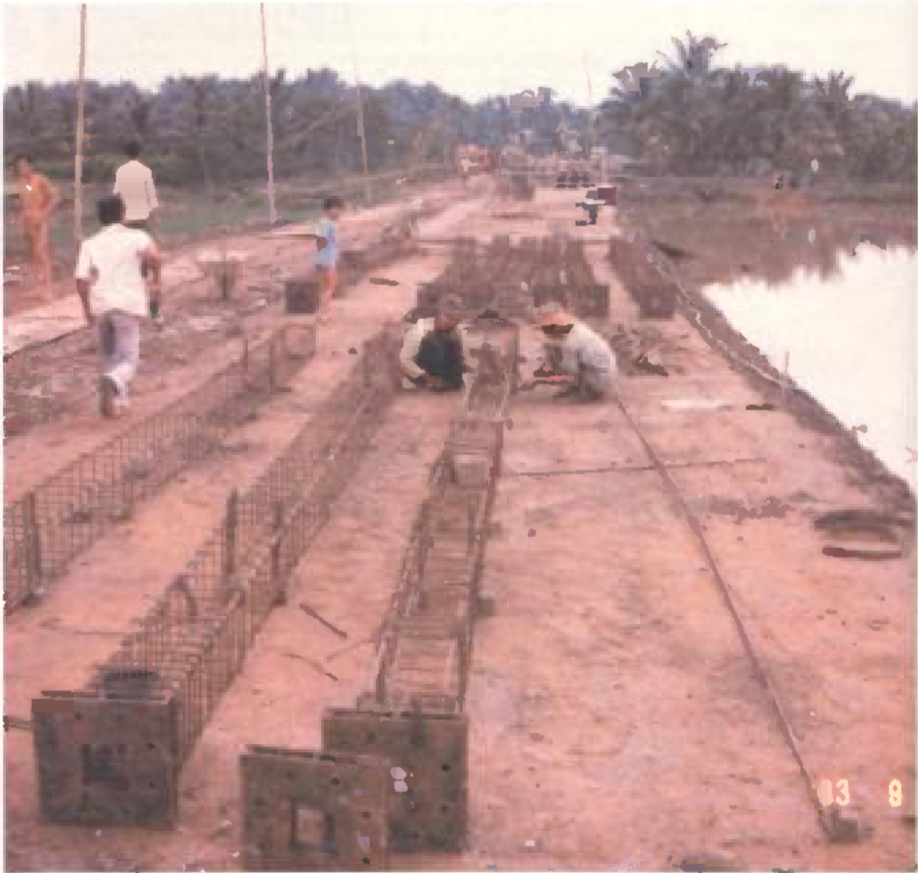
Concrete piling being prepared for the construction of the Hung My regulator
